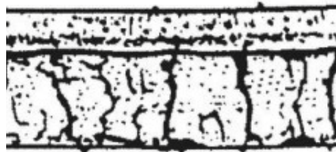
Belt showing signs of wear
